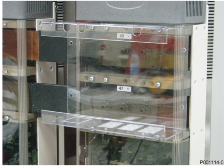
Figure 28: Cable raceway installed on the inverter module
